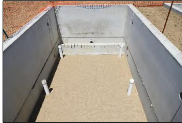
Sand filter chamber showing sand filter bed prior to installation. Credit: Ohio Department of Natural Resources Division of Soil & Water Resources.
