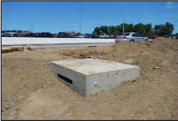
Sand filter installed to capture stormwater runoff from commercial parking lot . Credit: Ohio Department of Natural Resources Division of Soil & Water Resources.
