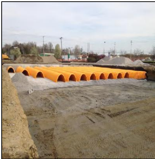
Open-bottom underground detention pipe segments awaiting installation into gravel backfilled storage layer. Credit: StormTech a Division of ADS, Inc.
