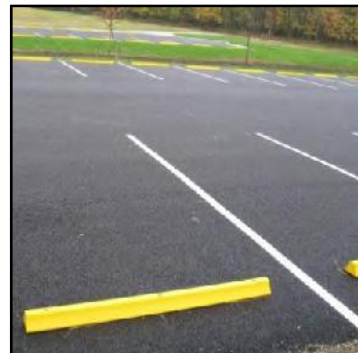
Porous asphalt within a parking lot. Credit: Chagrin River Watershed Partners, Inc.
