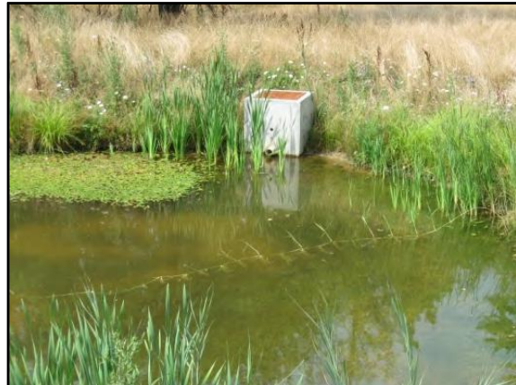
Outlet structure with multiple drains free of obstruction such as vegetation, trash or sediment. Credit: Summit Soil & Water Conservation District
