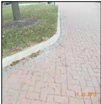
Permeable interlocking concrete pavement (PICP) shown with accumulated sediment along the curb indicating need for maintenance. Credit: Chagrin River Watershed Partners, Inc.
